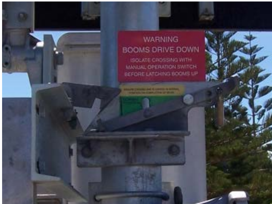
Figure 2015-1 Warning – Booms Drive Down sign.
