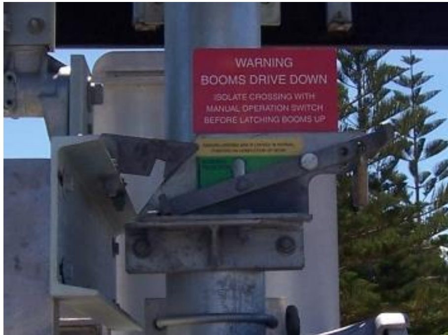
Figure 2015-1 Warning – Booms Drive Down sign.
